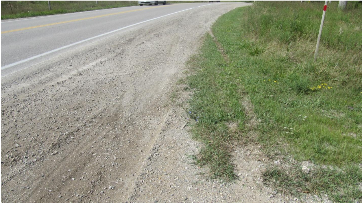
Figure 41: View, looking north, at the tire marks created on the east shoulder and roadside.
