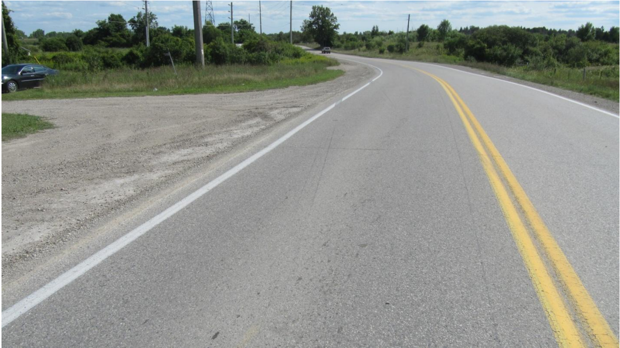
Figure 38: View, looking south, at the yaw marks in the northbound lane.
