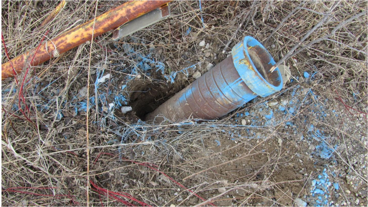
Figure 57: Close-up view of the flattened pipe and yellow pole that were struck by the southbound vehicle.
