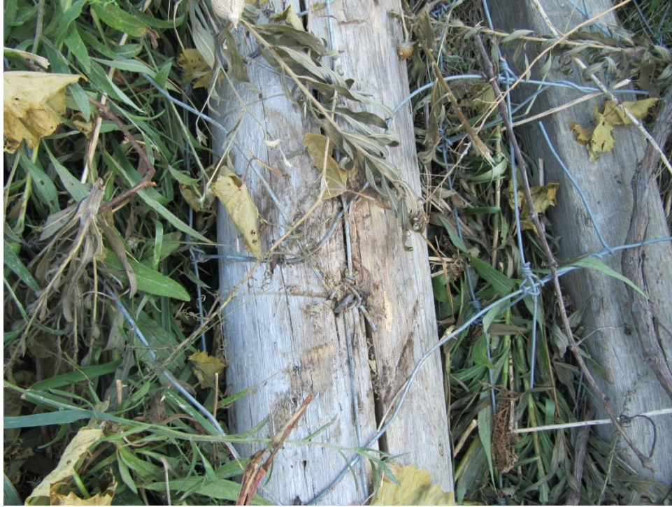
Figure 14: Close-up view of the fresh scrapes to one of the wooden posts cause by contact by the southbound vehicle.
