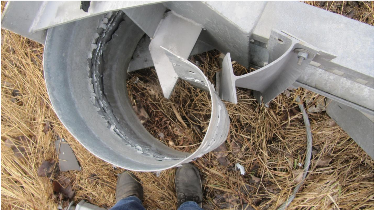
Figure 14: View, looking down, at the short length of guardrail that has passed through the throat of the ET-Plus terminal.
