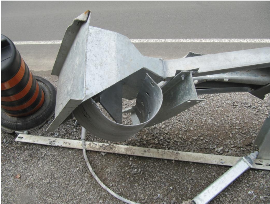
Figure 25: View showing that only a small length of the rail has passed through the throat of the terminal.
