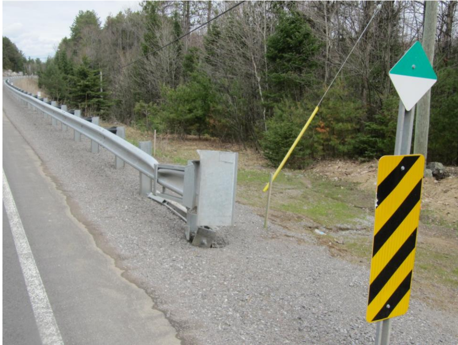
Figure 18: View, looking north, at the impacted ET-Plus terminal located on Highway 28. Note that there is very little evidence of damage yet there a major buckling of the guardrail just at the back of the terminal channel.
