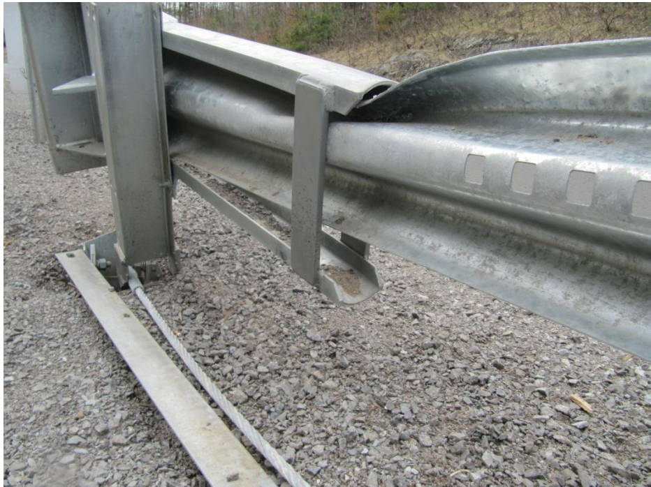
Figure 21: View of the rear edge of the terminal channel and the extent of the deformation to the top of the guardrail. The deformation of the rail prevents it from passing through the throat of the terminal and thus jamming which prevents the energy from being dissipated in the manner that is demonstrated in the controlled compliance tests.
