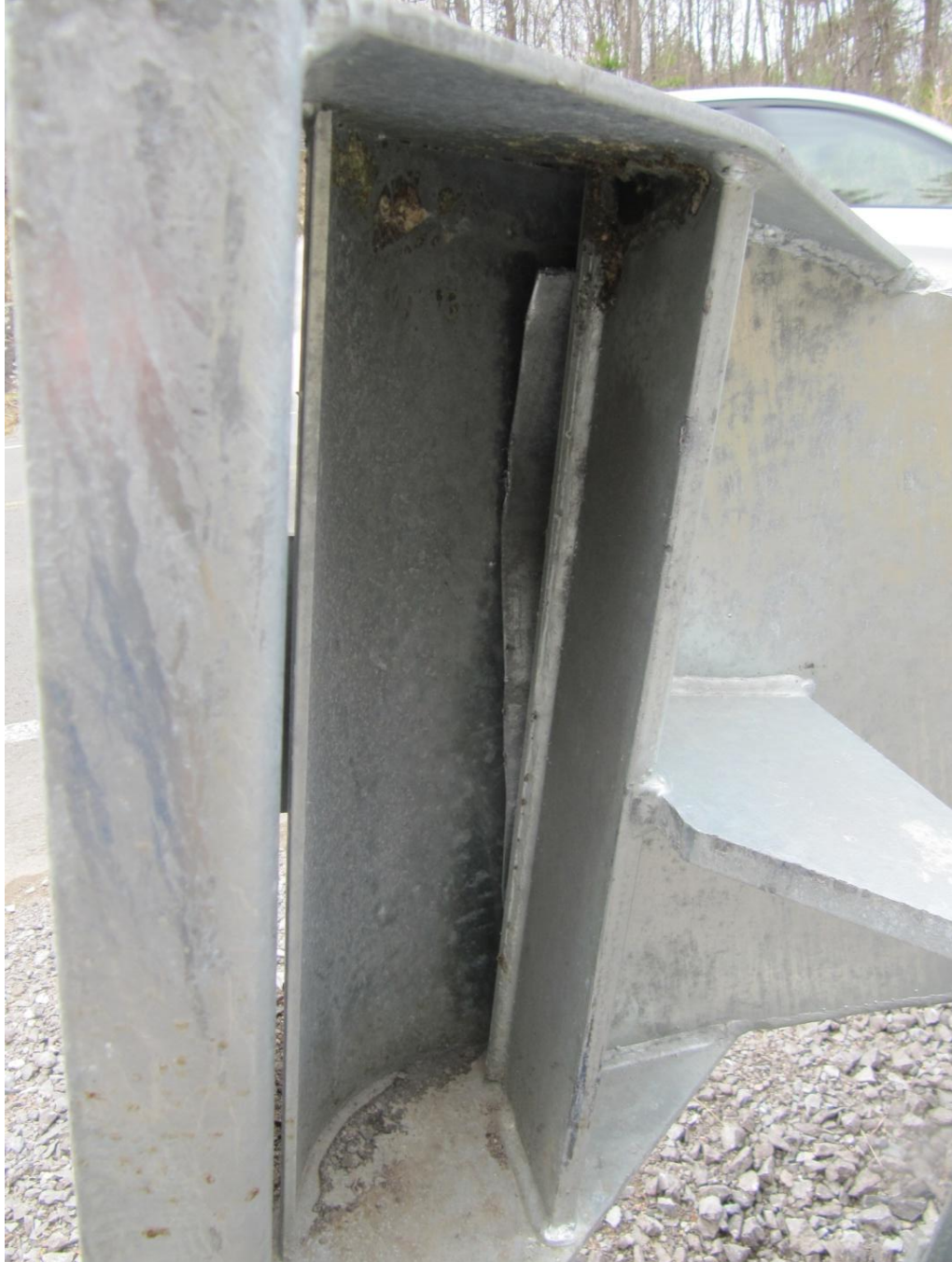
Figure 22: Close-up view of the throat of the terminal showing a very short portion of the leading edge of the rail beginning to be squeezed through the narrow throat. With the deformation of the top of the rail there is little hope that any additional length of rail will pass through this narrow opening and thus the designed method of energy dissipation has failed.
