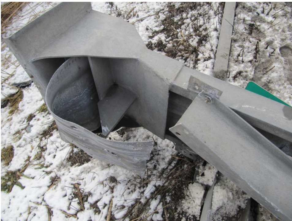
Figure 7: View looking down at the short length of rail that has been squeezed through the throat of the terminal. The flattening and coiling of the rail as it is squeezed through the narrow throat of the terminal is the mechanism that is shown to dissipate a large portion of the kinetic energy in controlled, compliance tests. Yet, in this real-life example that mechanism is largely nonfunctional.
