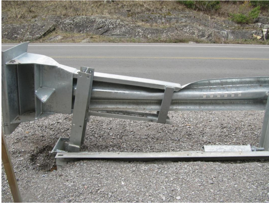
Figure 20: Ditch side view of the impacted terminal. This view illustrates the common manner in which the rear edge of the terminal channel impacts the top edge of the rail causing the rail's deformation.
