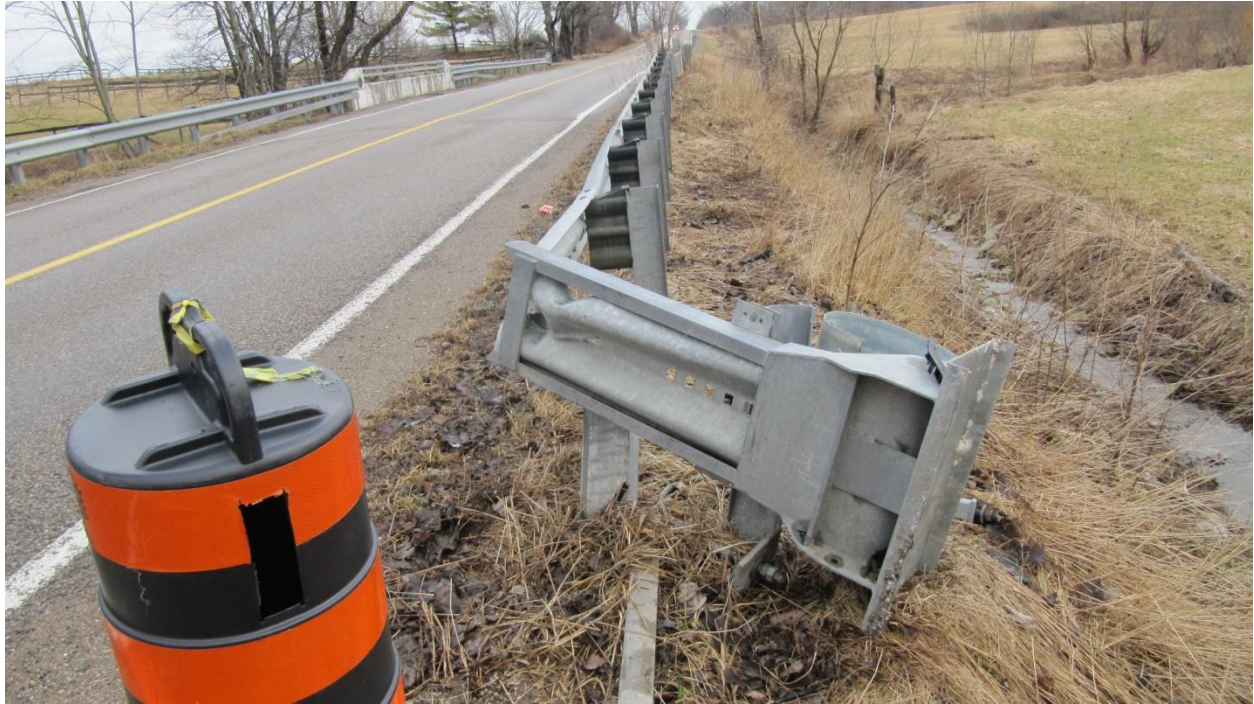
Figure 11: View, looking south, at the ET-Plus terminal which has been rotated allow to a ninety degree angle with respect to the length of the guardrail.
