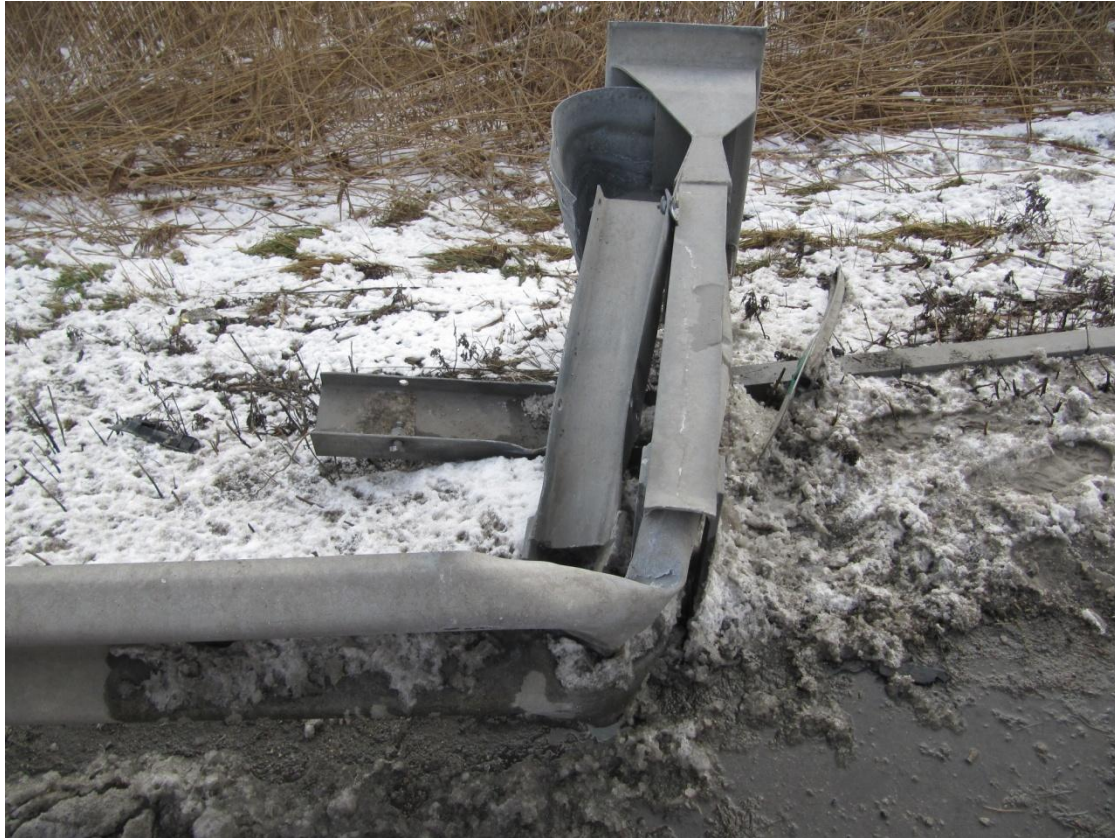
Figure 8: View showing how the terminal has rotated to a ninety degree angle with respect to the guardrail. Clearly no additional length of the rail could be expected to pass through the terminal.
