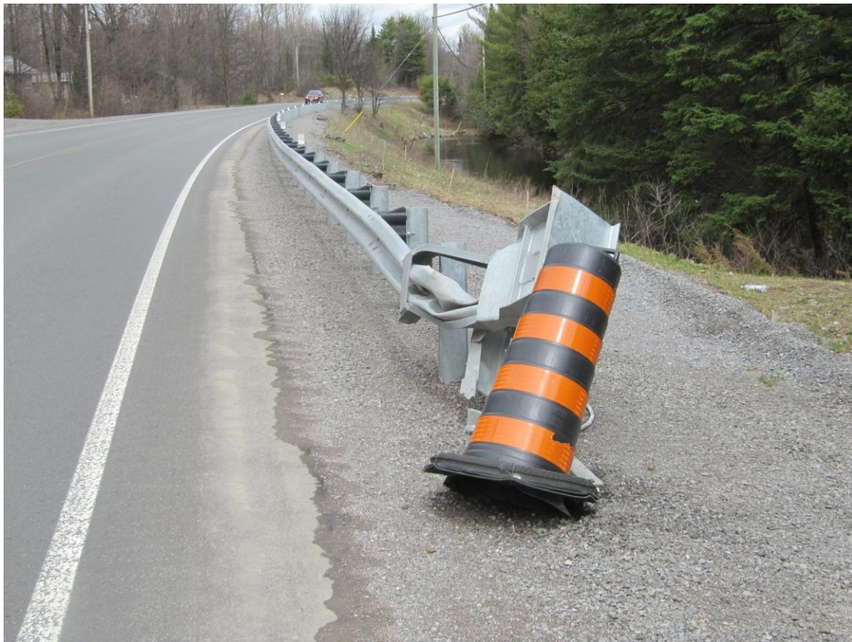
Figure 23: View, looking north at the damaged ET-Plus terminal on the east side of Highway 28.
