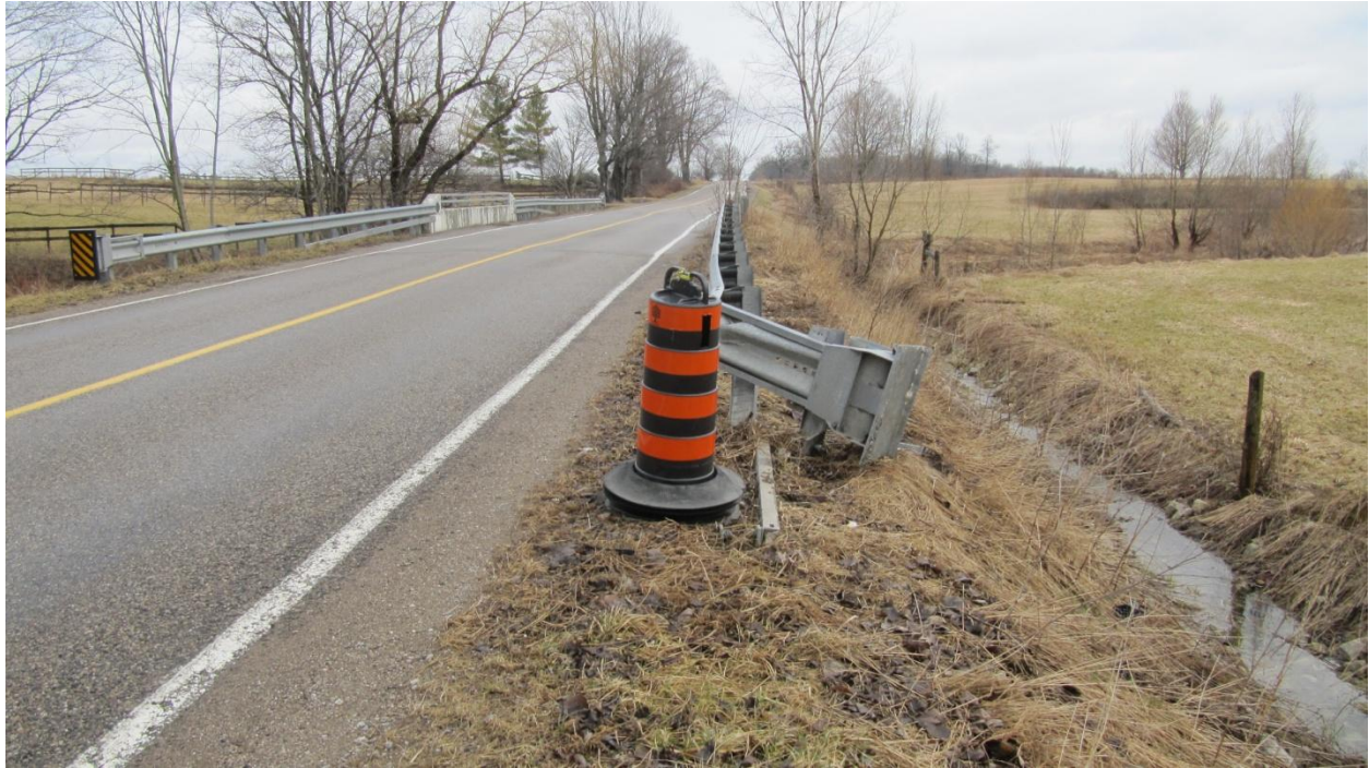
Figure 9: View looking south at the struck ET-Plus terminal on the west side of Wonderland Road.
