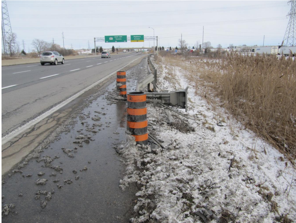
Figure 1: View, looking east, at the damaged ET-Plus terminal located on the south side of the eastbound lanes of Highway 401 just west of Highbury Avenue.
