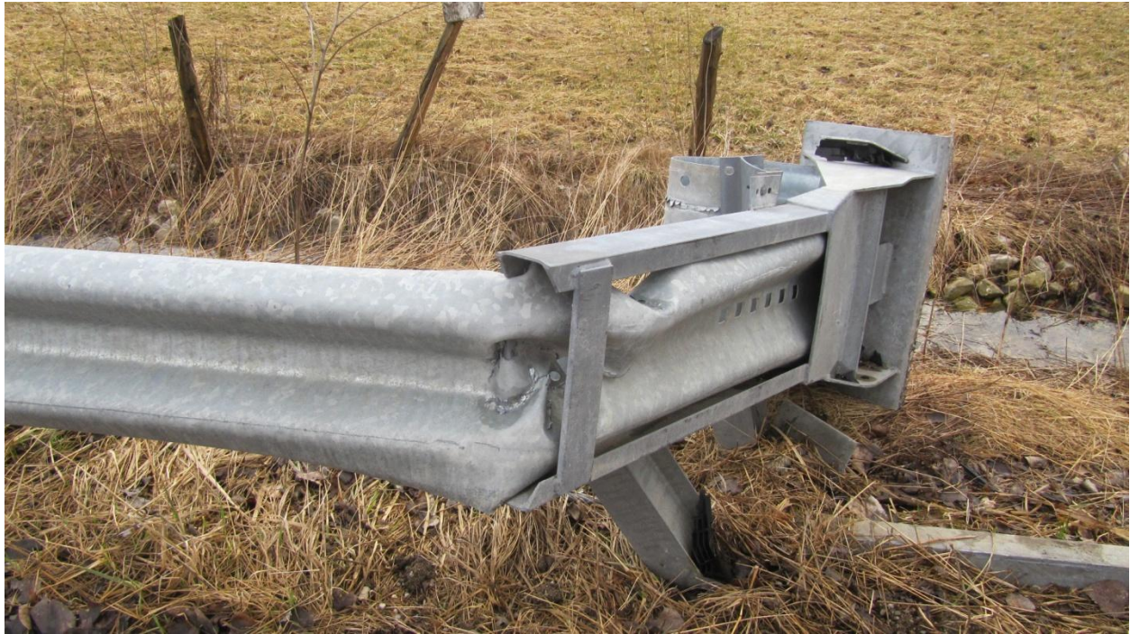
Figure 12: A view of the location at the back of the ET-Plus terminal where the guardrail has buckled thus not allowing any additional length to be squeezed through the throat of the terminal.
