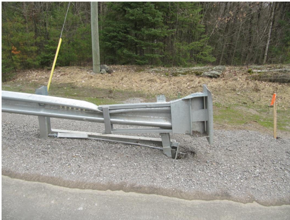
Figure 19: View of the impacted terminal showing that the plate has been rotated upward while the rear of the channel has been rotated downward onto the top edge of the guardrail causing the significant deformation in the rail.
