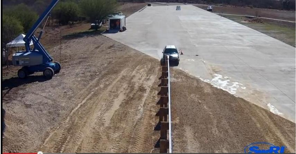
Figure 28: Example of the compliance test set-up taken from the South West Research Institute's (Texas) re-testing of the ET-Plus in early 2015.
