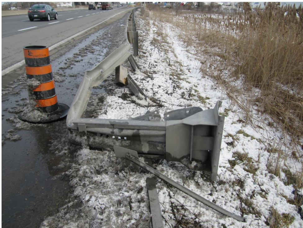
Figure 2: View looking east at the ET-Plus terminal showing it has rotated to a ninety degree angle as the guardrail has buckled and prevented passage through the throat of the terminal.
