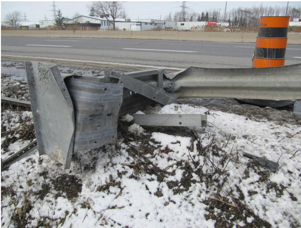
Figure 5: View of the ditch side of the terminal showing the short length of the rail that passed through the throat thus demonstrating the small amount of energy that was dissipated by this mechanism.
