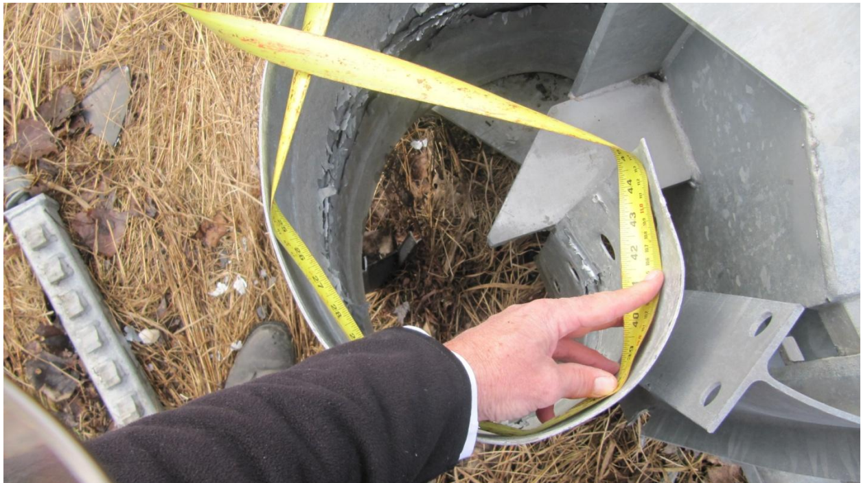
Figure 16: View of the measurement tape being wound around the contours of the deformed rail that has passed through the throat of the ET-Plus terminal.
