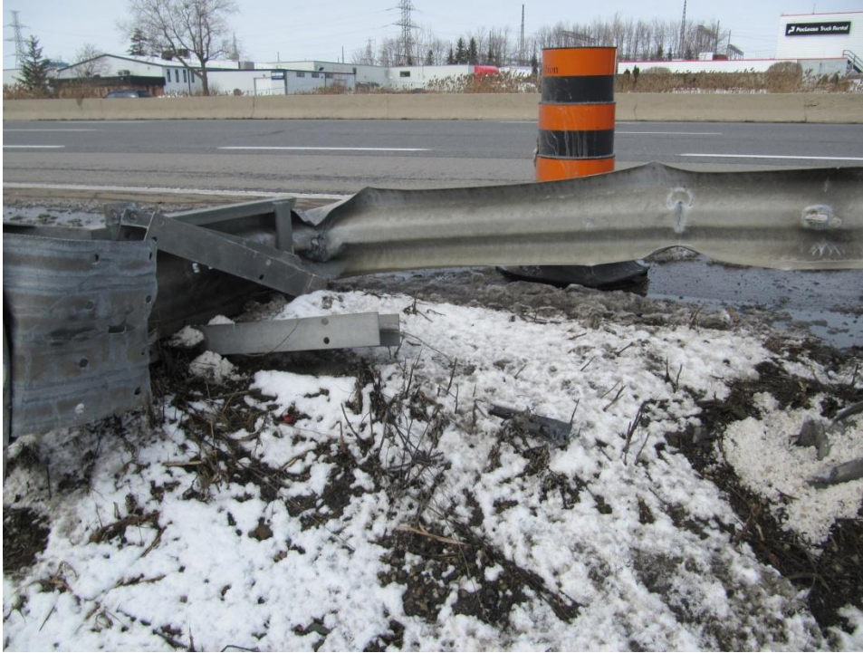
Figure 6: View showing the portion of the rail just behind the rear edge of the terminal. An obvious downward buckling of the rail exists at the rear of the terminal demonstrating that no additional length of rail would pass through the terminal.
