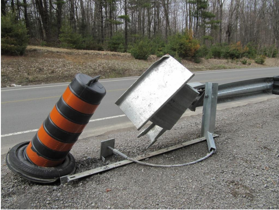
Figure 24: View showing that the terminal plate has been rotated upwards.
