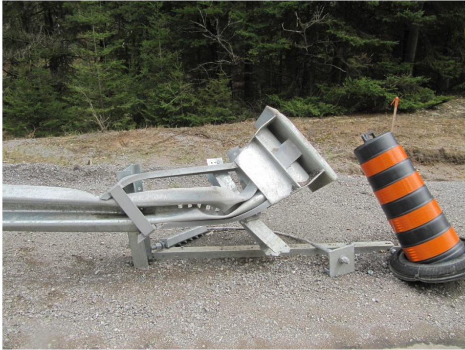
Figure 26: This view shows how the channel has been greatly deformed along with the rail within it.
