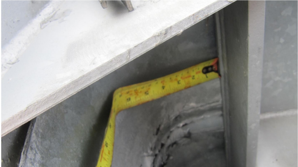
Figure 15: View showing the method used to measure the length fo the guardrail that has passed through the throat of the terminal. Here the zero end of a tape measure is placed at the throat and the tape is then wrapped around the coil of the deformed rail as shown in Figure 16.
