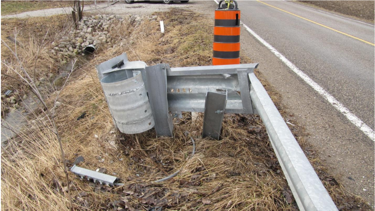
Figure 13: View, looking north, at the ET-Plus terminal which has been rotated almost ninety degrees preventing any further riding of the terminal along the rail and thus preventing any further energy dissipation by this mechanism.
