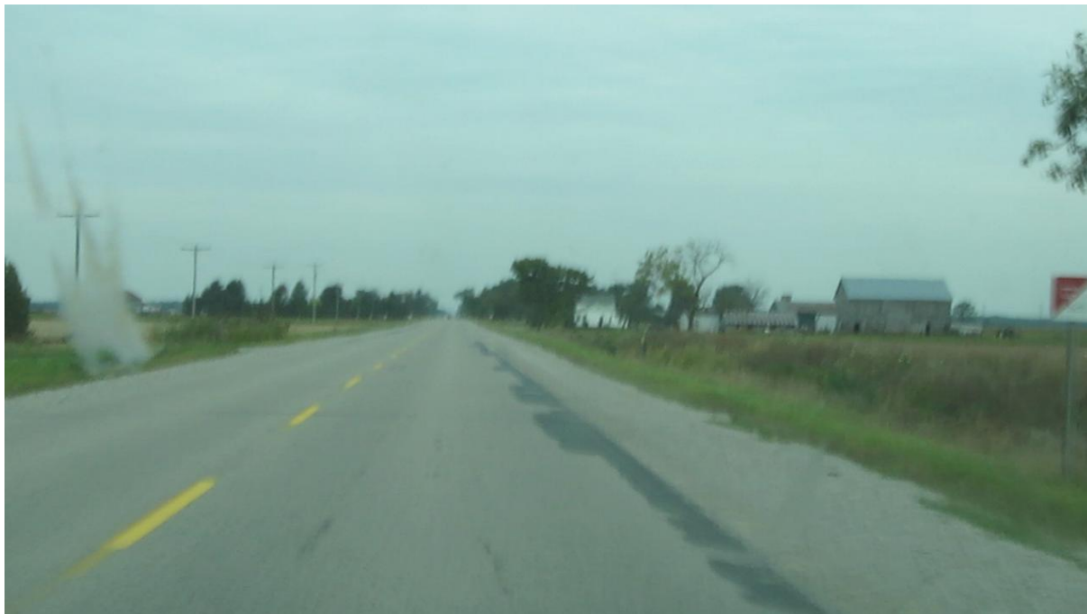
Figure 3: Out of focus view caused by the vibration of our vehicle travelling over one of the lateral cracks in the pavement.
