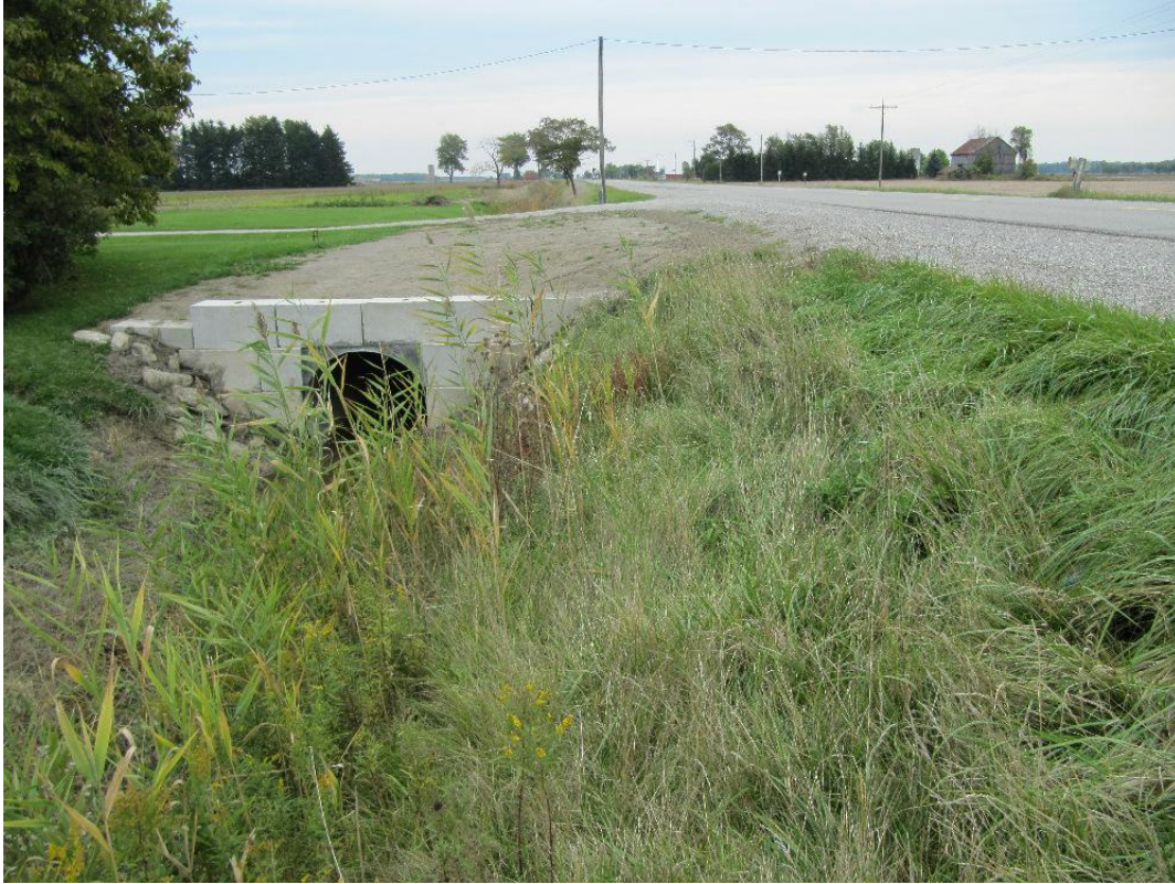
Figure 7: Eastward view of north ditch and a source of standing water that is hidden by tall grasses.
