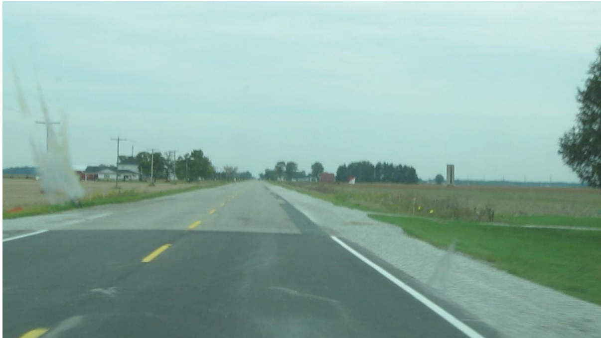
Figure 2: View of end of new paving of Courtright Line just west of Black Ash Road.
