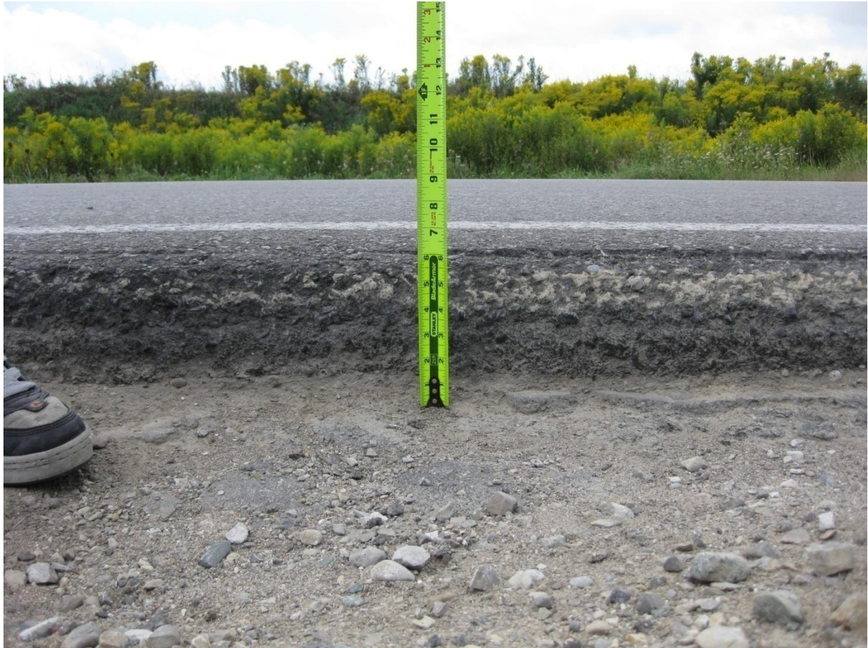
Figure 2: Example of a dangerous edge drop-off
