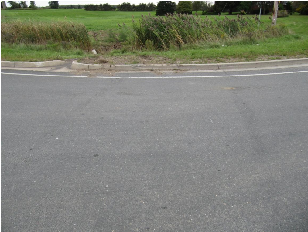
4-View, looking southwest toward the exit location where one of the vehicles entered the ditch
