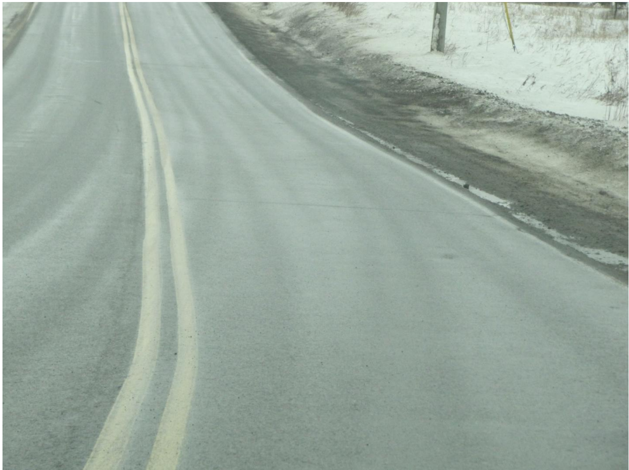
Figure 7: View, looking north near the north curve showing the road conditions on January 31 st . The condition of the right snow bank can be compared to the same location from February 2 nd in Figure 8 to demonstrate that a snowplow plowed the snow sometime between those dates.
