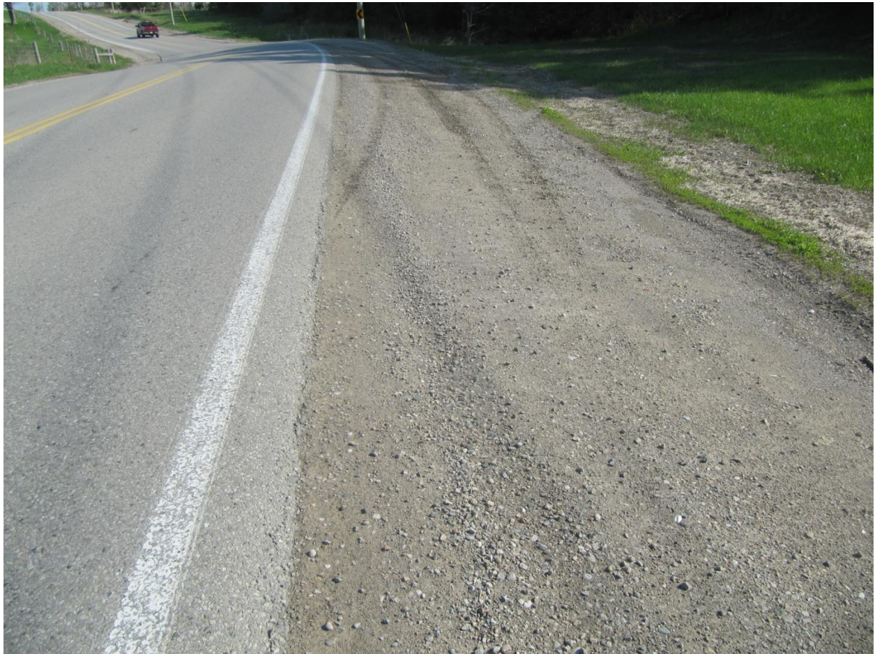
Figure 34: Incident documented on May 19th, 2014. This is a view looking north along the east shoulder between the two curves of the S-Curve. Yaw marks in the shoulder show that a southbound vehicle rotated clockwise as it approached the camera. The driver regained control in the foreground thus the yaw marks are no longer visible.
