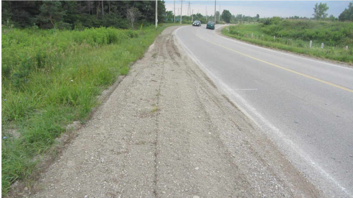
Figure 39: Incident documented on August 5th, 2014. This is a view looking south along the east shoulder at the north curve. Yaw marks from as northbound vehicle can be seen in the shoulder as the vehicle began to rotate counter-clockwise. The tire marks show the vehicle returning to the road surface in the foreground as it continues its rotation.
