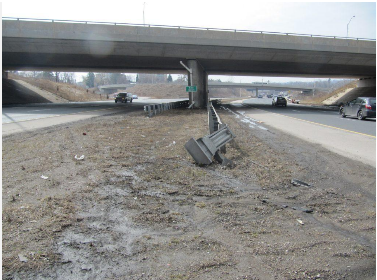
An impacted ET-Plus terminal at the end of the guardrail on Red Hill Valley Parkway near Queenston demonstrates that not all barriers in a median will perform as intended and expected.
