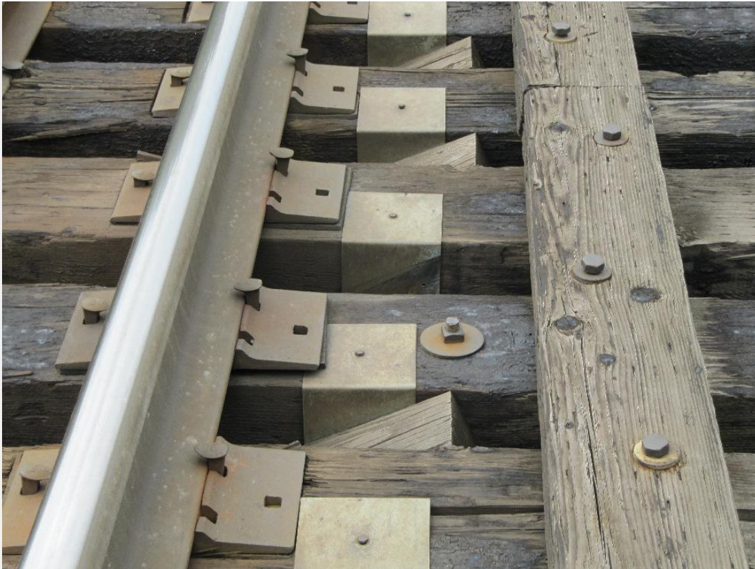
Closer view of missing “spacer” between the railway ties of the CP rail truss spanning Western Road in London.
