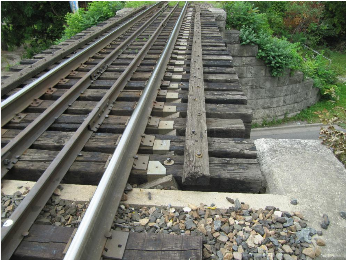
View upon climbing onto the CP rail truss on August 28, 2013 to explore why and how the wood had fallen.
