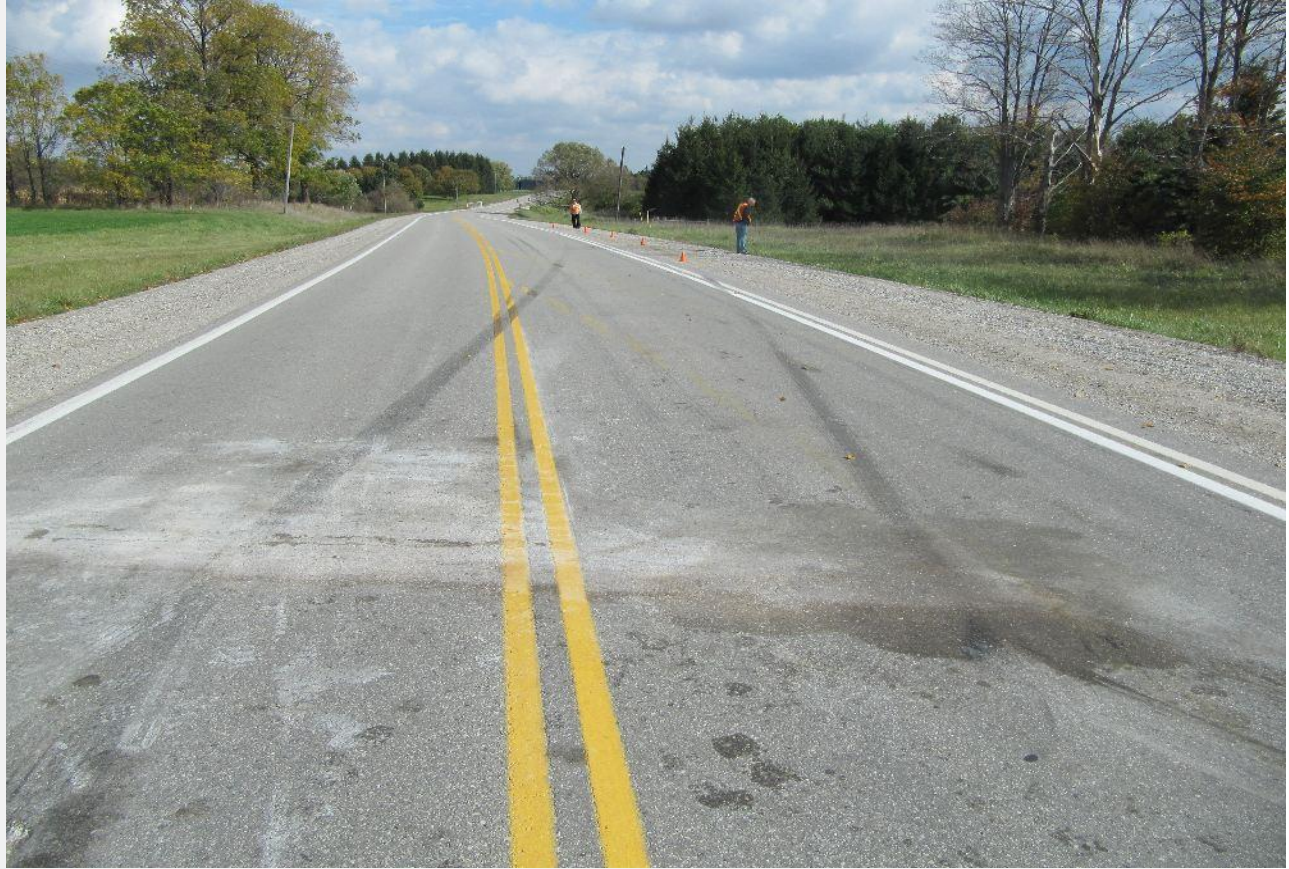
View, looking east along Road 88, from just west of the area of impact. the curve and pre-crash tire marks on the shoulders are located in the background.
